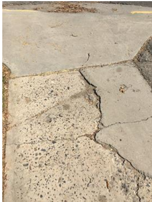
Figure 3: Cracked sidewalks present tripping hazards.
