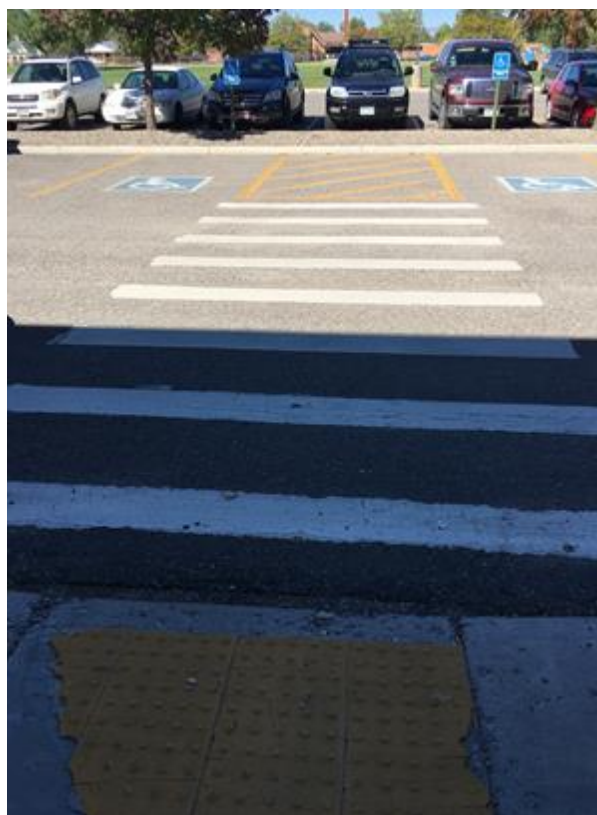
Figure 1: Handicap ramp is not accessible from parking lot; truncated dome pad may be a tripping hazard.
