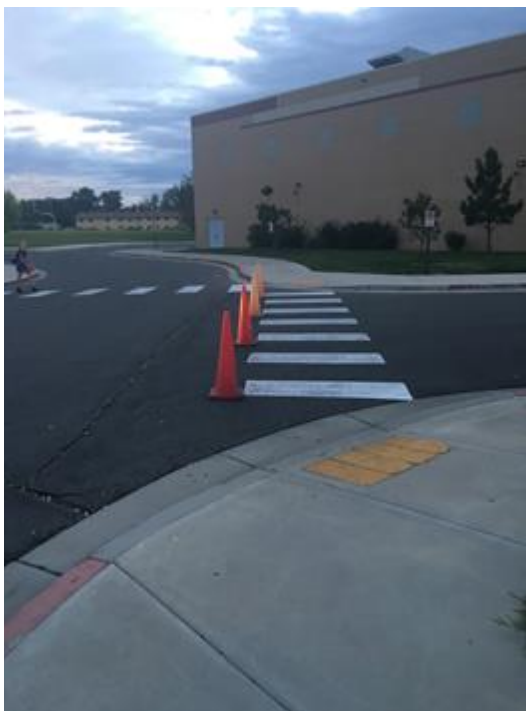
Figure 1: Cones are used to block off bus unloading/loading zone. Also, the truncated dome strips are peeling and need to be replaced in the ramp.
